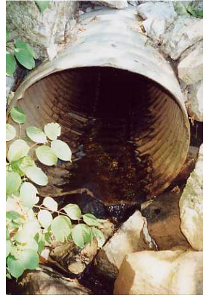
Concord wishes to improve the quality of storm water discharges
